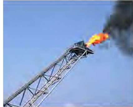
Darflare™ heat shield installed on the Chevron Benchamas platform, Thailand.
