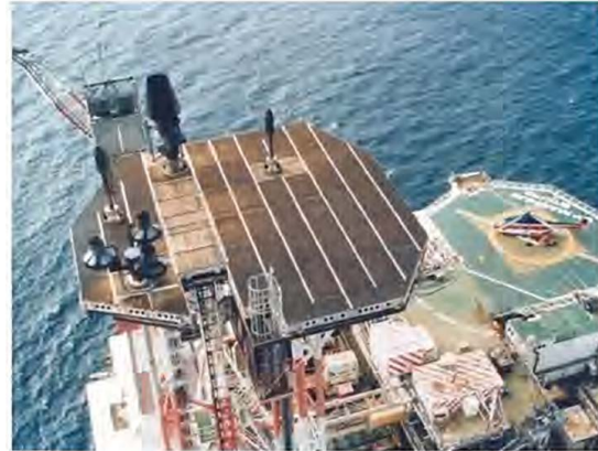
Darflare™ 'chevron' system installed on the BP Magnus Platform, UK North Sea
